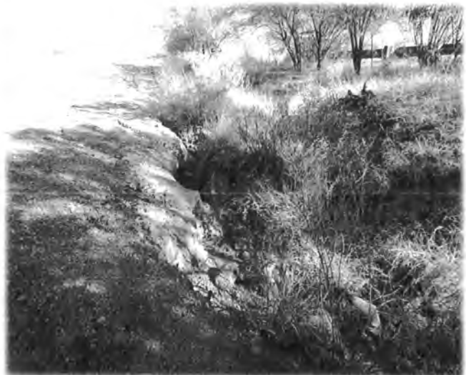
PHOTOGRAPH NO. 14 Deep erosion rills located along the south inspection road. Viewed from the west.
