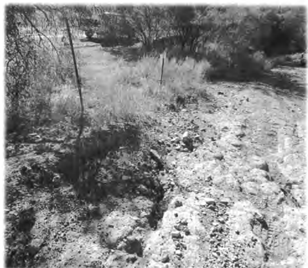
PHOTOGRAPH NO. 16 Deep erosion rills located along the south inspection road. Viewed from the east.
