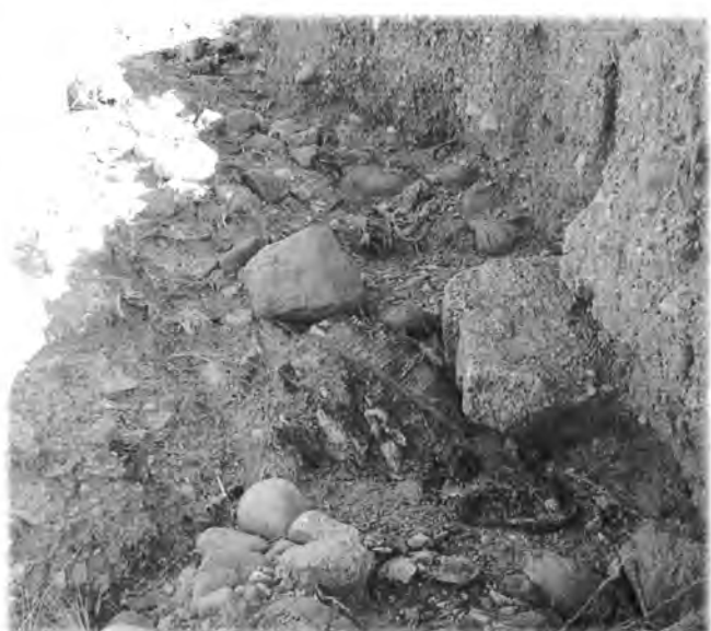
PHOTOGRAPH NO. 24 Deep erosion rills located along the on the west slope. Viewed from the west.
