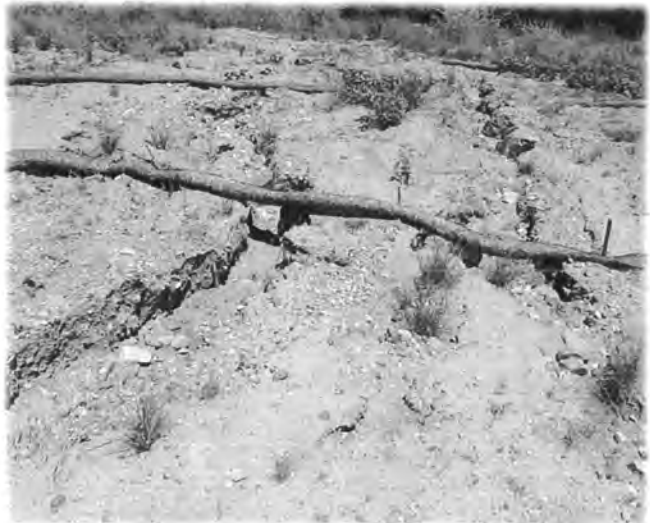
PHOTOGRAPH NO. 6 Erosion rills located on west slope. Viewed from the north.
