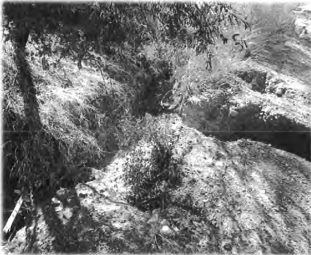
PHOTOGRAPH NO. 13 Deep erosion rills located along the south inspection road. Viewed from the east.
