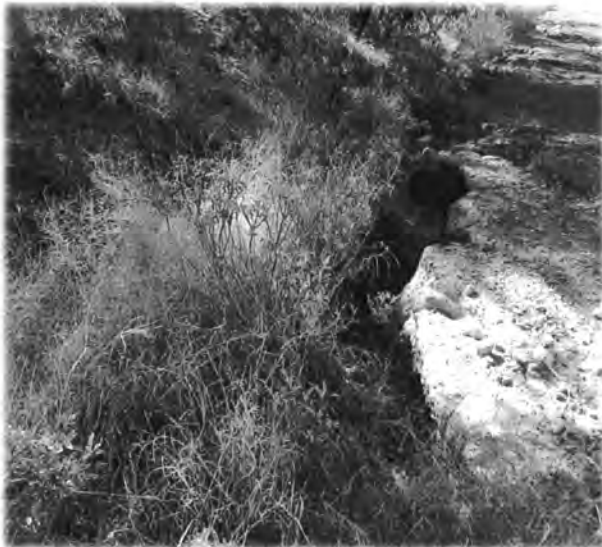
PHOTOGRAPH NO. 15 Deep erosion rills located along the south inspection road. Viewed from the north.
