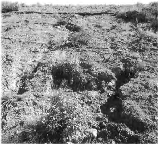
PHOTOGRAPH NO. 11 Erosion rills parallel to the west spillway. Viewed from the North.
