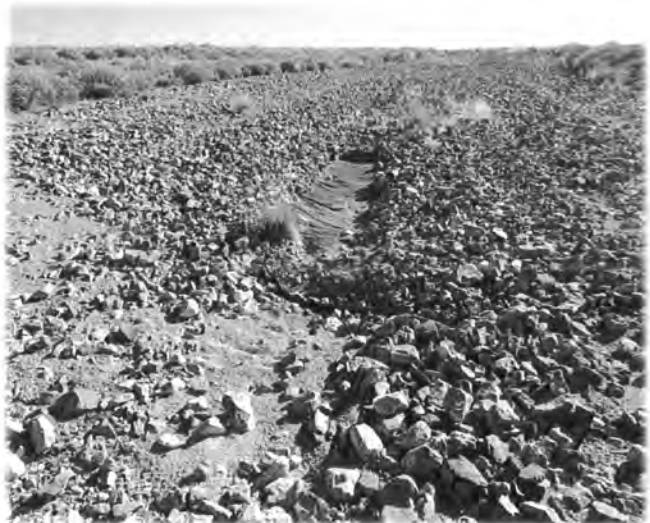
PHOTOGRAPH NO. 10 Exposed silt covered fabric located on north spillway. Viewed from the North.
