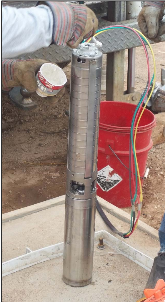
Grundfos MS402 Pump with 1.5 Hp motor. Intake set at 326.4 feet bls.
