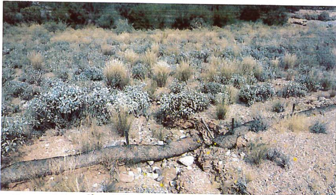
Photo 12: Erosion rill on south slope of landfill
