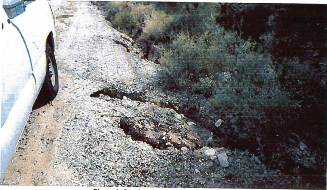
Photo 1: Erosion on south perimeter road
