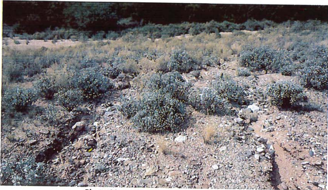
Photo 11: Erosion rill on north slope of landfill
