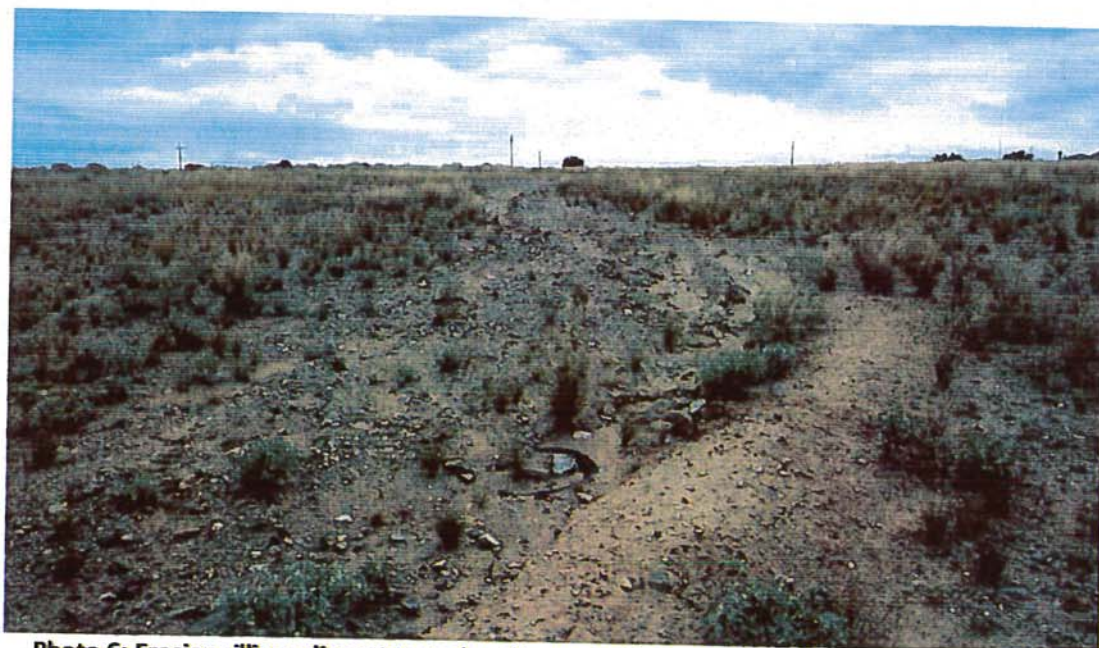
Photo 6: Erosion rilling adjacent to rock spillway, north central landfill cap, note exposed tire
