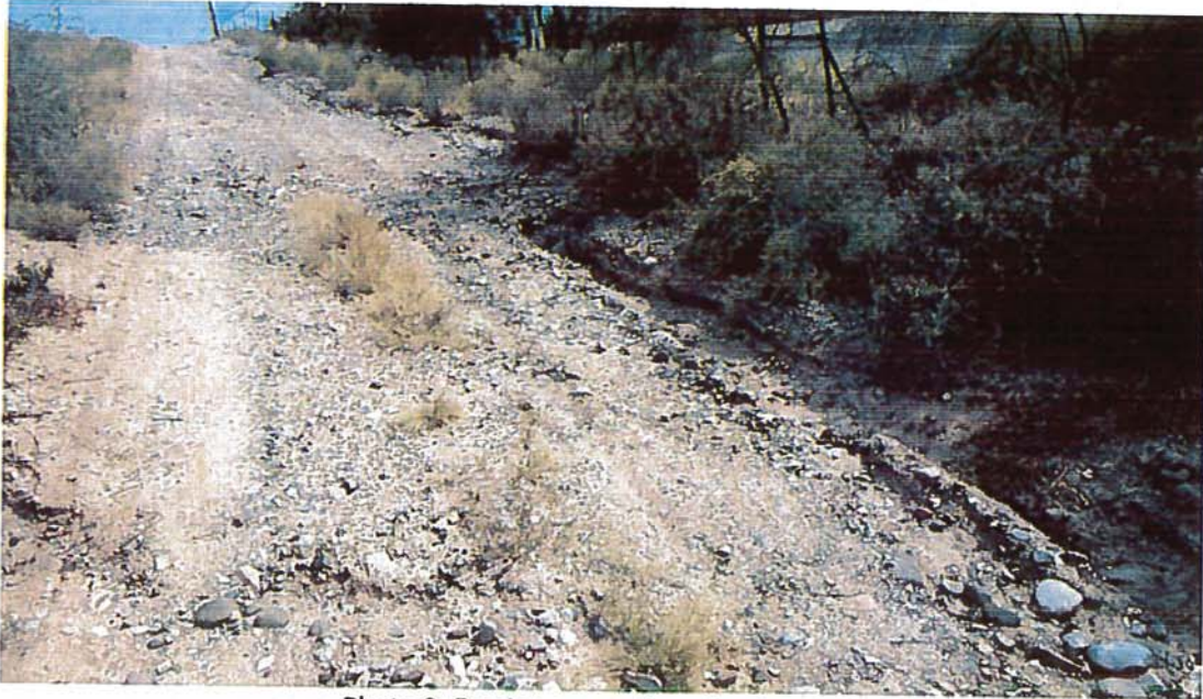
Photo 3: Erosion on south perimeter road
