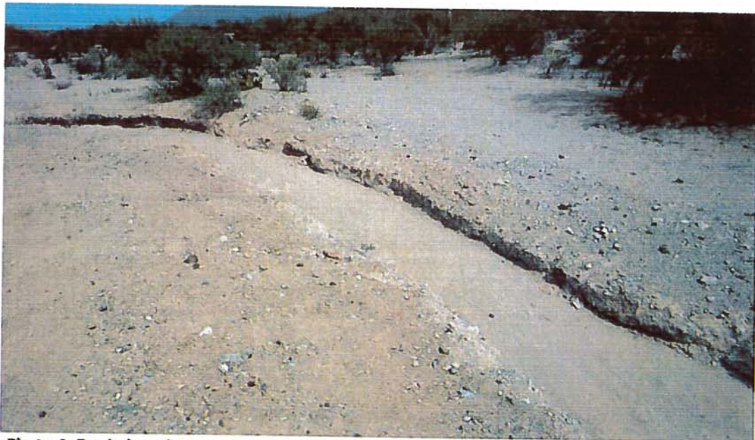
Photo 4: Eroded road connecting wells WR-385A & WR-385B with wells WR-448A & WR-448B
