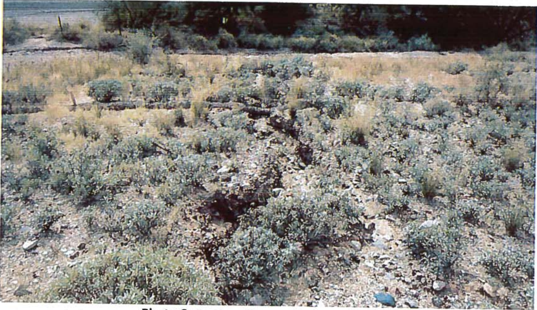
Photo 9: Erosion rill on south slope of landfill
