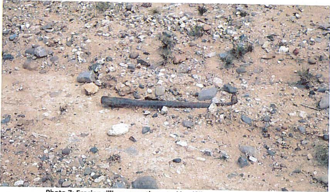
Photo 7: Erosion rilling on north central landfill cap, note exposed pipe
