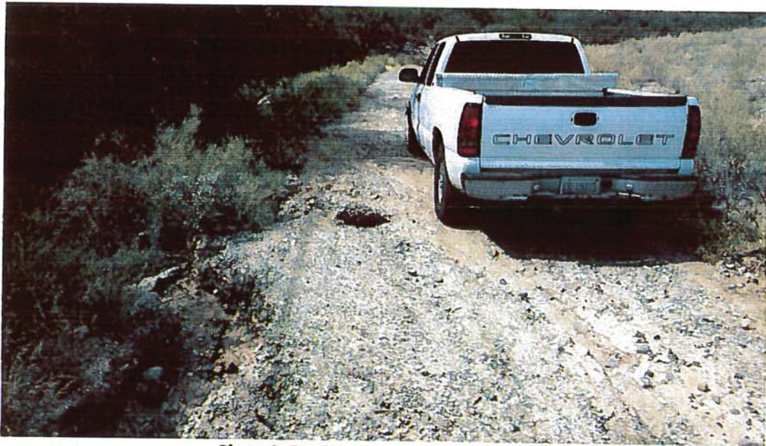
Photo 2: Erosion on south perimeter road
