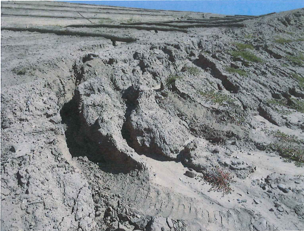
Photo 3: Erosion at upstream (south) end of landfill west slope (at river)
