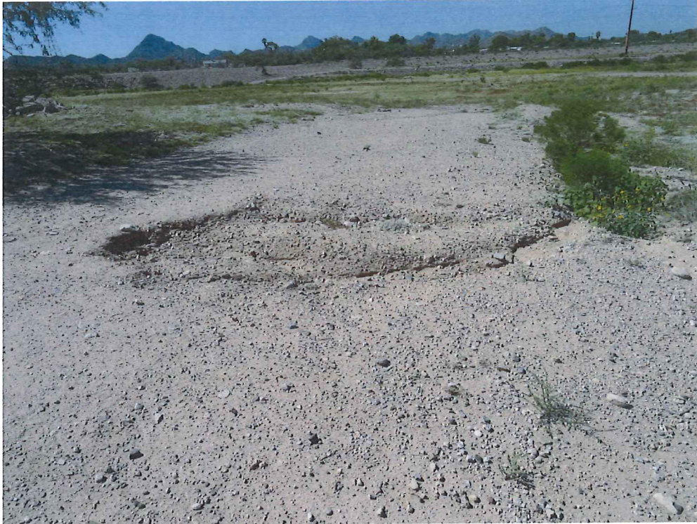
Photo 1: View of erosion & head cutting on north inspection road
