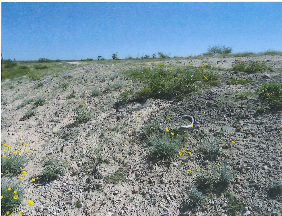
Photo 6: Miscellaneous debris outcropping on landfill slope
