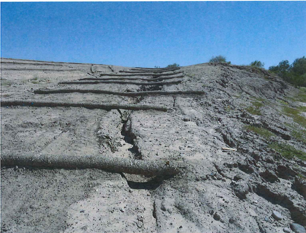
Photo 4: Erosion at upstream (south) end of landfill west slope (at river)
