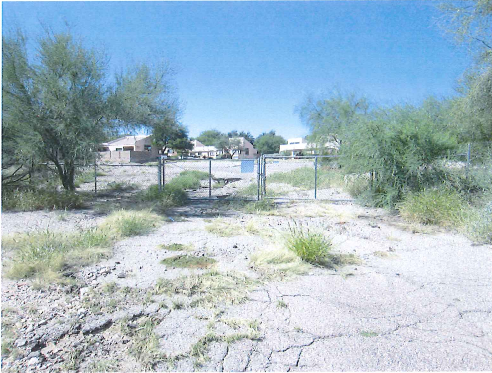
Photo 1: Damaged asphalt drainage
