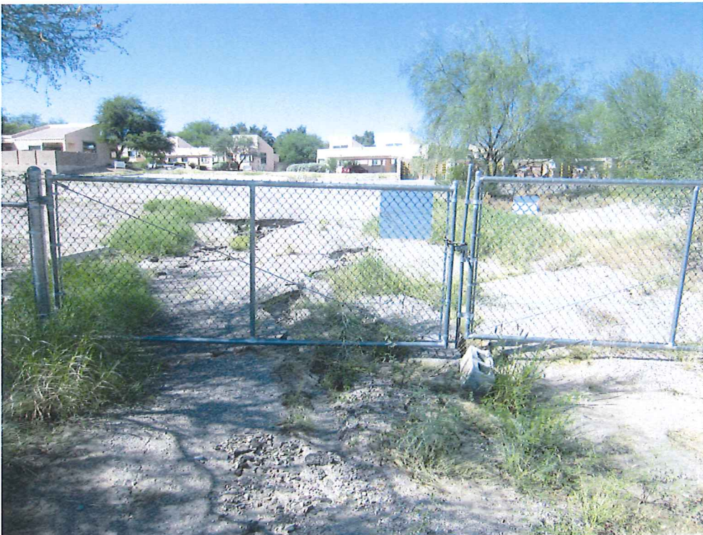
Photo 2: Western portion of damaged asphalt drainage
