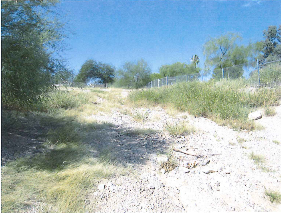
Photo 3: Rilling on earthen drainage, worst rilling obscured by weeds
