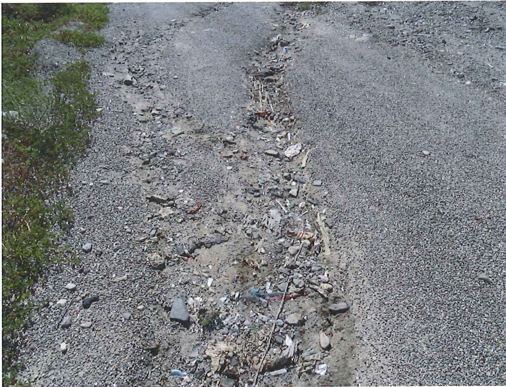
Photo 2: Exposed trash in rills in inspection road
