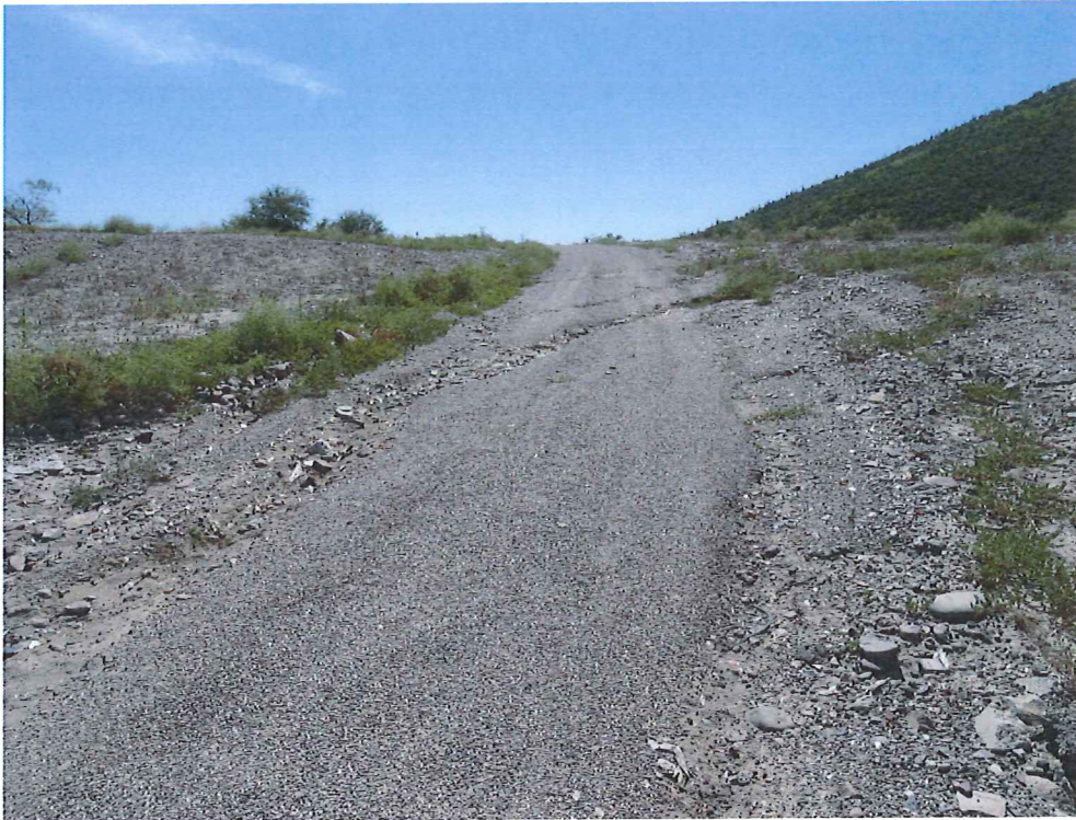
Photo 1: Erosion rills on inspection road with exposed trash, view to the south
