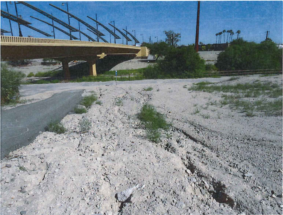
Photo 2: Erosion rilling on east slope of Congress LF near the Cushing Street Bridge
